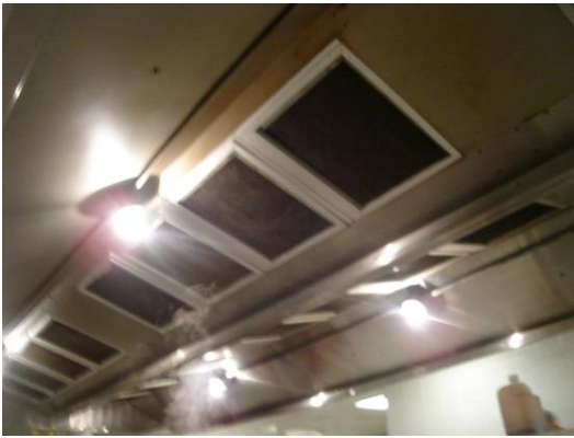
Extractor, Cocina, Incendio.
